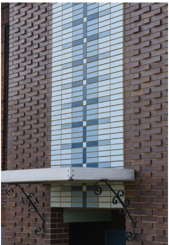
Fig. 15. Wall fragment from the Holy Cross Church in Dayton (OH), 1964, architect Jonas Mulokas [from authors private archive]
