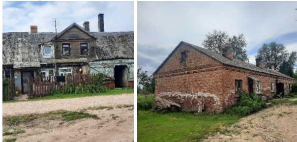
Fig. 15, 16. Villages Progress, Spartaks. Workers' house was adapted to a multi-apartment building in the post-war years [photos by A.Ziemeļniece, 2024]
