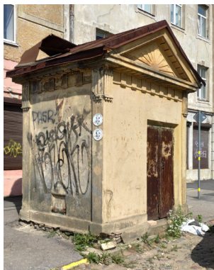
Fig. 18. Small transformer substation, typical design, at the corner of Latgales iela and Katoļu iela. 1922–1929
