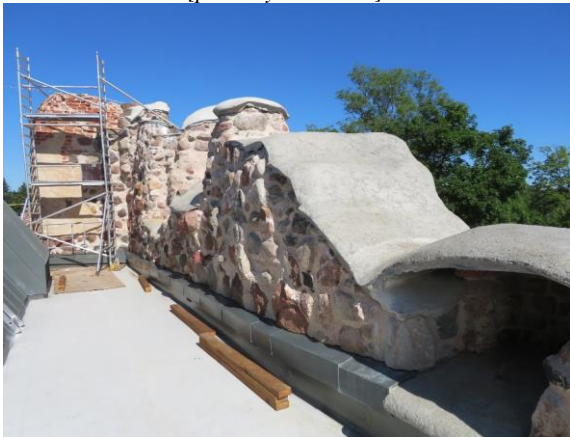
Fig. 10. Coverage of the upper part of walls with fibro-concrete [photo by the author]
