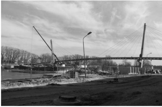
Fig. 8. Jelgava. The reconstruction boulevard promenade and new bridge by Driksa (2012) [Source: photo by the author]
