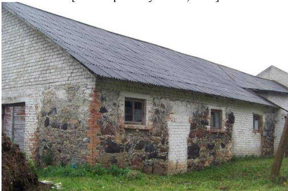
Fig. 7. The fragments of the building from the 80s of the 19 th century are supplemented with the silicate brick masonry in the 60s of the 20 th century. The former stockyard at Kulpju Manor, Jaunsvirlauka Parish [Source: photo by author, 2013]
